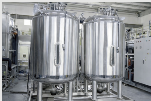
External CIP water tank
